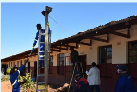
Lecturers and students of the Waterberg TVET College Engineering and Skills Training Centre, made sorely needed repairs to the lighting in the school yard
