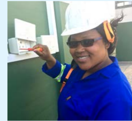
Noluphiwa Gcele from Miya Electrical demonstrates the installation of an outdoor socket
