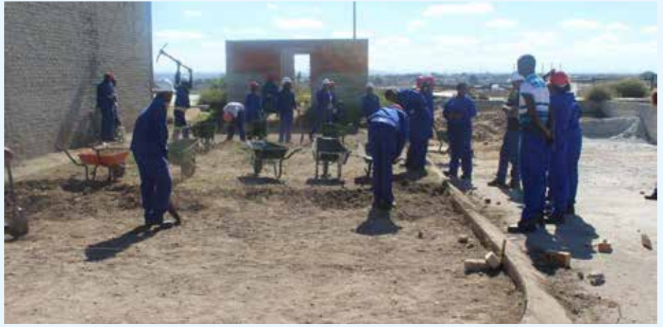
Civil Engineering Students beautify the face of Port Elizabeth TVET College Iqhayiya Campus and gain valuable, certified Work Based Experience in the process
